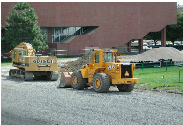
The outdoor track is being widened to 8 lanes and surfaced with Mondo 14mm Super X Performance.
